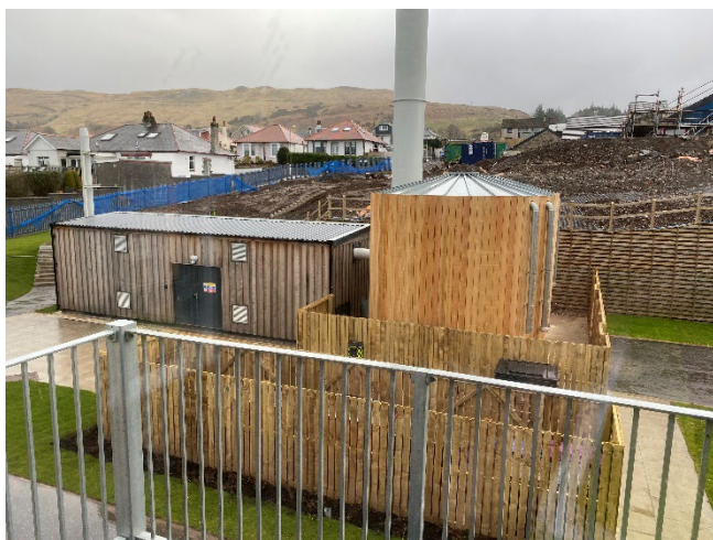
Biomass District Heating Network at Flatt Road, Largs
